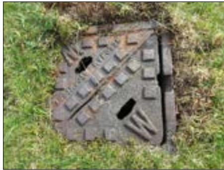
Figure 70: FID6 - Drain cover on route of water pipeline, Settlebeck Gill.
