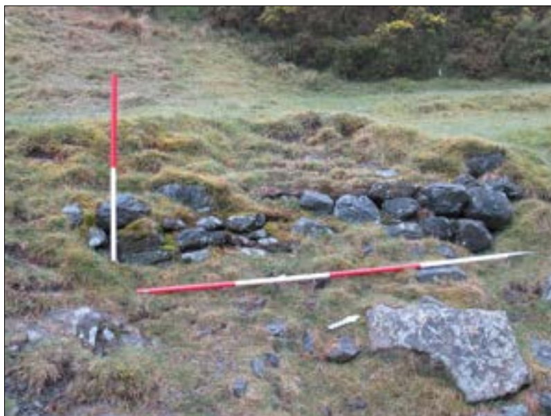
Figure 71: FID7 - Revetment wall supporting a trackway containing a pipe outlet, Settlebeck Gill.
