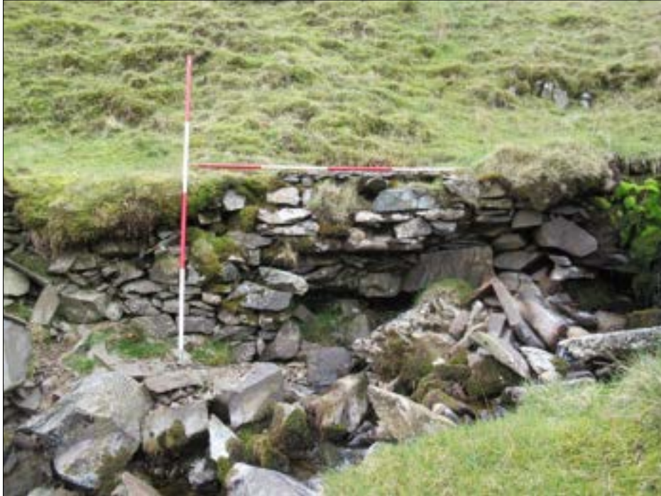
Figure 65: FID2 - Revetment wall with pipe outlet, chamber and trackway behind, Ashbeck Gill.
