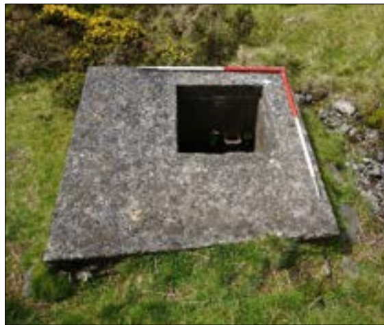
Figure 87: FID34 - Concrete chamber forming part of the former water supply for Sedbergh Town, facing west.
